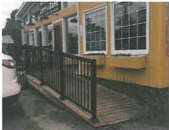
Figure 3.1: Accessibility ramps with handrails allow individuals to access businesses barrier-free – Cobden, Ontario.
